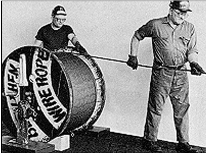
The wire rope reel is mounted on a shaft supported by jacks. This permits the reel to rotate freely, and the rope can be unwound either manually or by a powered mechanism.
